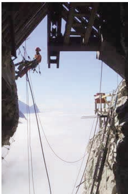
Re-installing the Black Angel cable car. One of the blasters is preparing charges before blasting another slice of rock at the upper terminal of the cable car (600m above fjord level). The view of the fjords below is obstructed by low-lying clouds. Courtesy: Angus & Ross plc.
