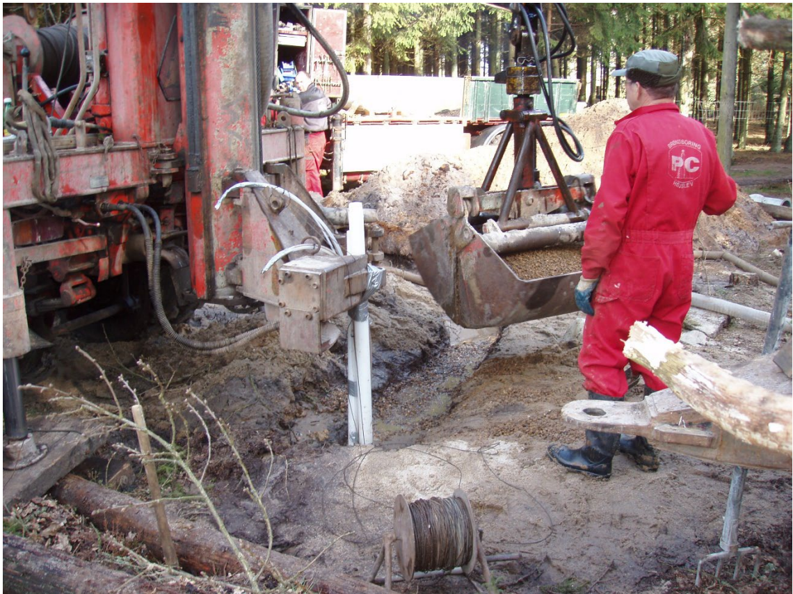
Figure 1. Well completion. In this case, there are two casing strings in the same borehole.
