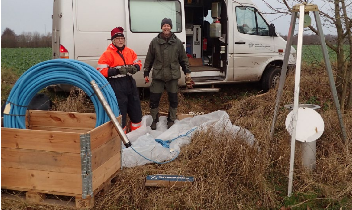
Figure 7. Preparation for installation of a larger electric submersible pump and hoses. The equipment is pre-assembled in the workshop, where hose lengths are adjusted to the technical completion of the borehole.
