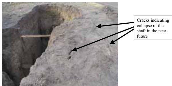
Figure 7. Cracks near a shaft. These cracks indicate that there will be cave in of the walls in the near future.
